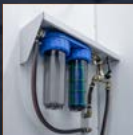
WASTEWATER FILTRATION Integrated two-stage wastewater filtration system
