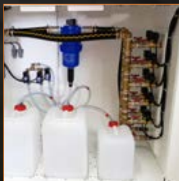
Automatic disinfectant dosing system
